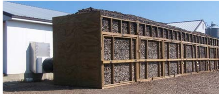
Researchers at the University of Minnesota have tested a vertical biofilter that treats exhaust air from a commercial-type pig nursery barn. Exhaust air flows from the barn through ducts and then into a tall, packed bed of living material that biologically degrades the pollutants in the exhaust air. Photo by Larry Jacobson, University of Minnesota.
